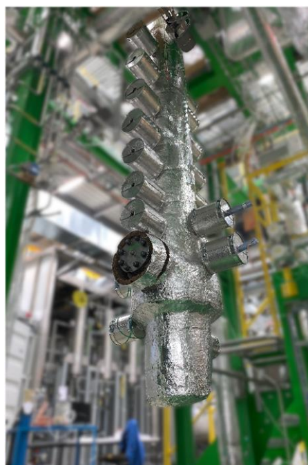
Figure 1 Reactor of the pilot plant for bubbling fluidized bed methanation
